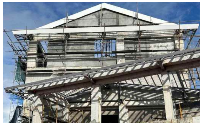
Roofing on the fourth floor was already being installed during the visit.
